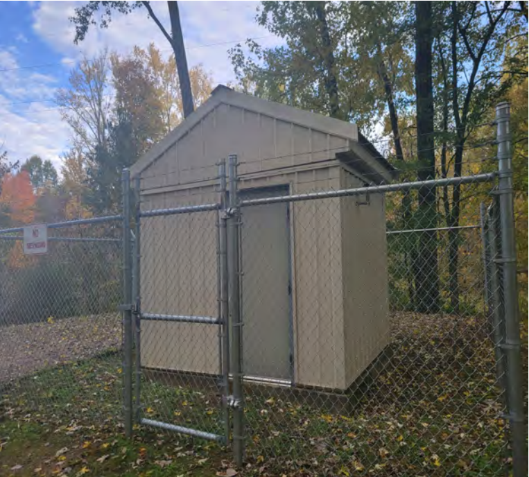
NOTES: Includes: 15hp pump, controls, and SCADA.
