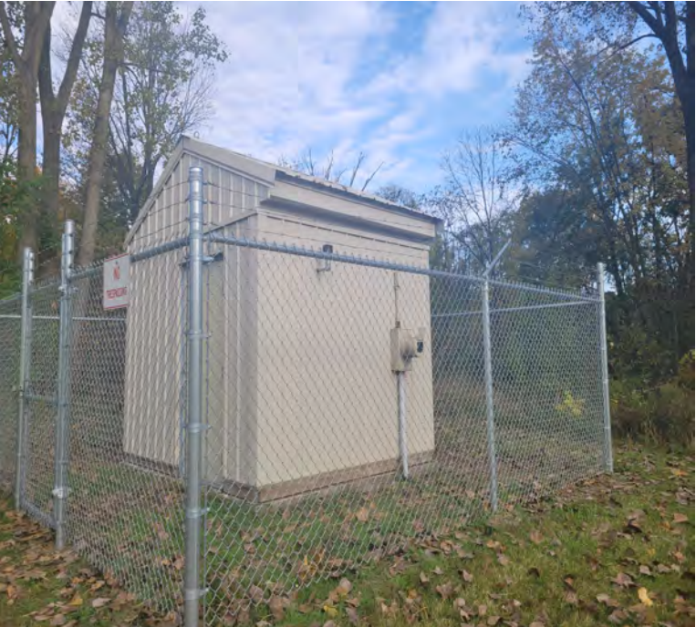
NOTES: Includes: 15hp pump, controls, and SCADA.
