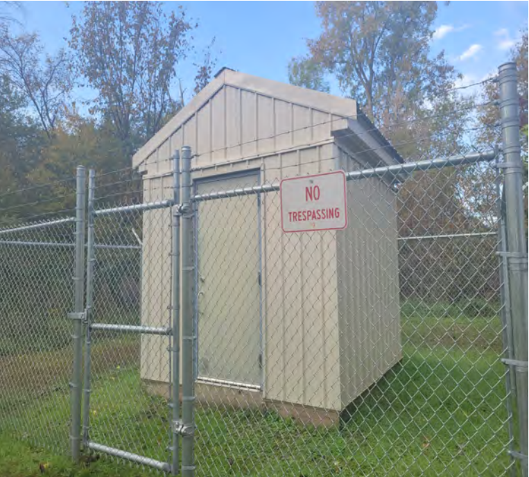
NOTES: Includes: 15hp pump, controls, and SCADA.
